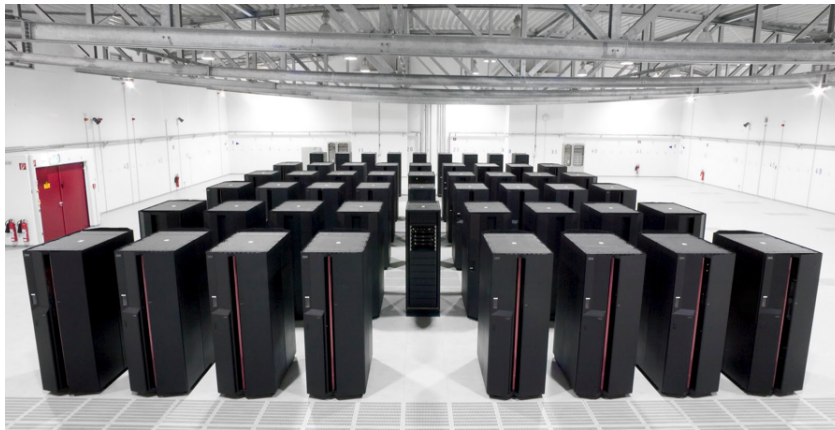
Figure 4.9: Picture of the Blue Waters Supercomputer inside its building.
